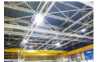
High-ceiling LED lighting
