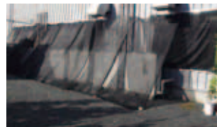
Shading of air conditioner outdoor units
